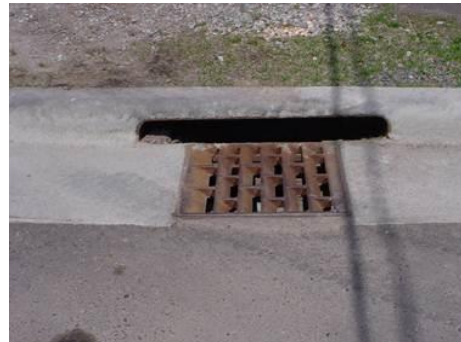
Storm Sewer - Catch Basin
