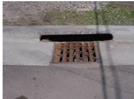
Storm Sewer - Catch Basin
